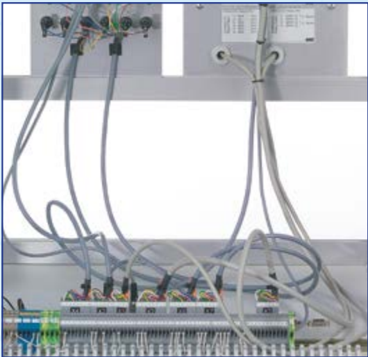
Industry-standard, flexible cabling
