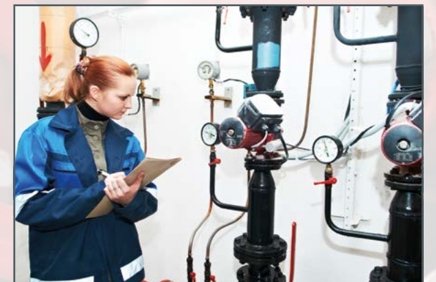
Checking the system components
