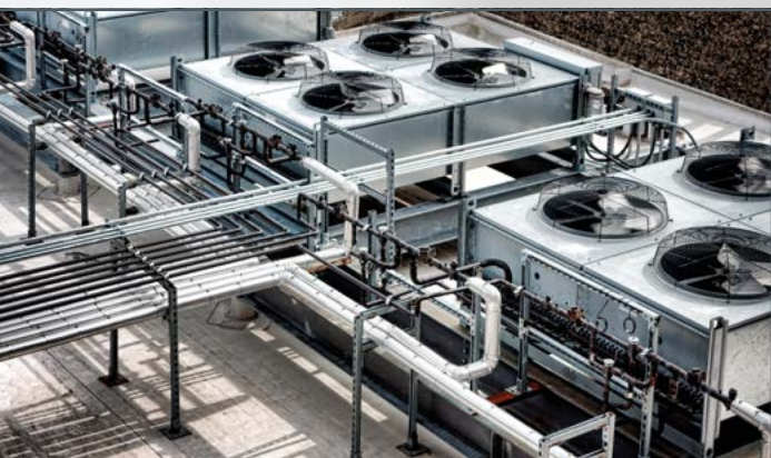
Condenser in a refrigerant network
