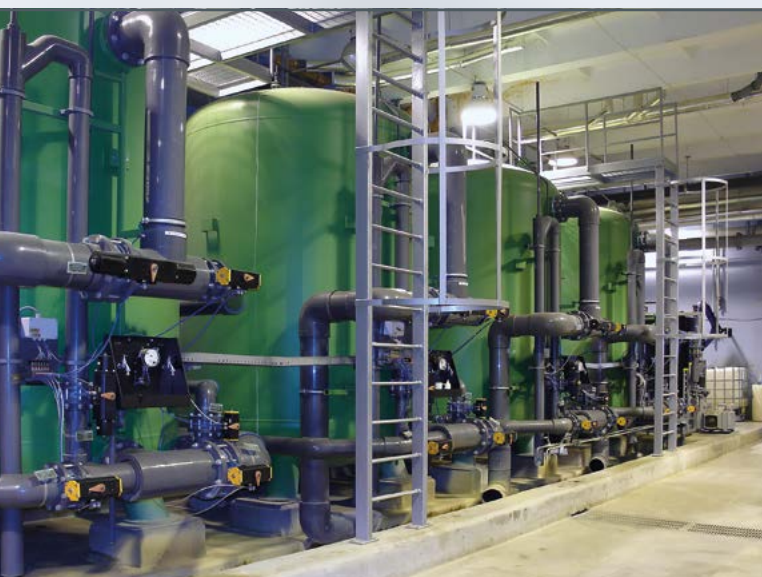
Continuous-flow adsorber in a water treatment plant
